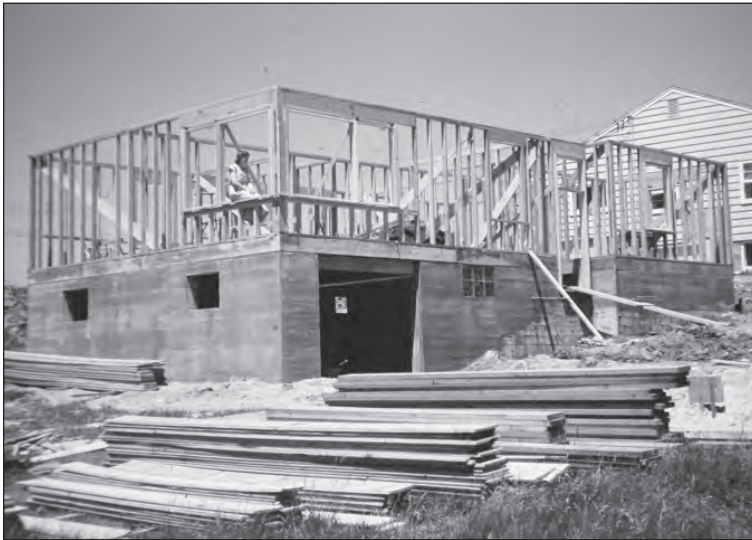
The Saeman’s house at 564 Gately Terrace under construction in 1950. Ronnie Saeman shown sitting in window.
