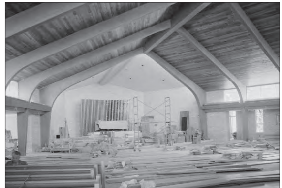
Interior view of Our Lady Queen of Peace church while still under construction in 1955.
