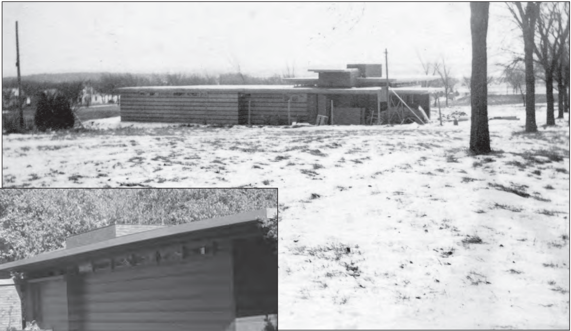
The Jacobs' Usonian Home under construction in 1936 (WHi 25625) and present view in 2009.
