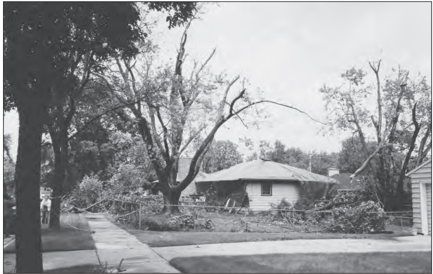
The house at 4321 S. Owen Drive shows roof damage from the tornado.
