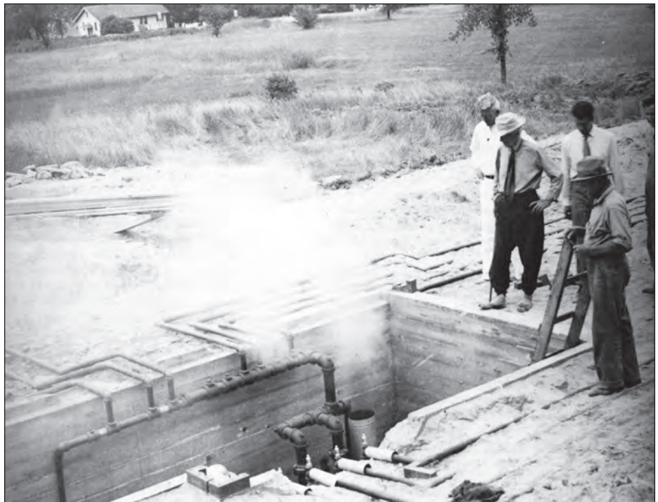
Frank Lloyd Wright inspecting the heating system of the Usonian Home at 441 Toepfer Avenue in 1936. (Photo from the Jacobs family collection.)
